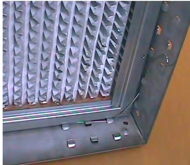
FIG. 4-25 – FULLY INSTALLED FILTER
