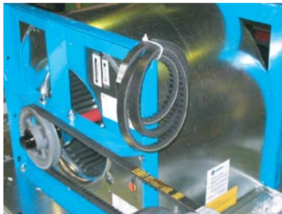
SPARE FAN BELT (Attached to Fan)
