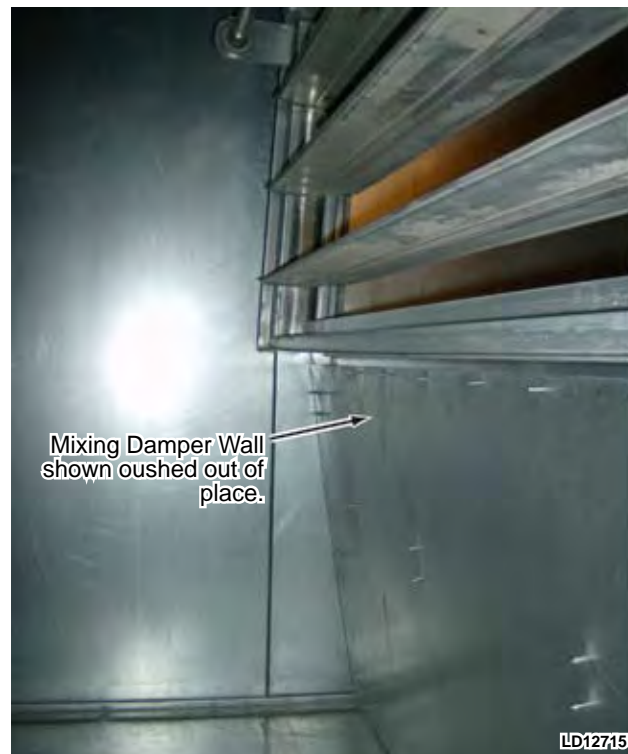
FIG. 5-119 – MIXING DAMPER WALL PUSHED OUT OF PLACE
