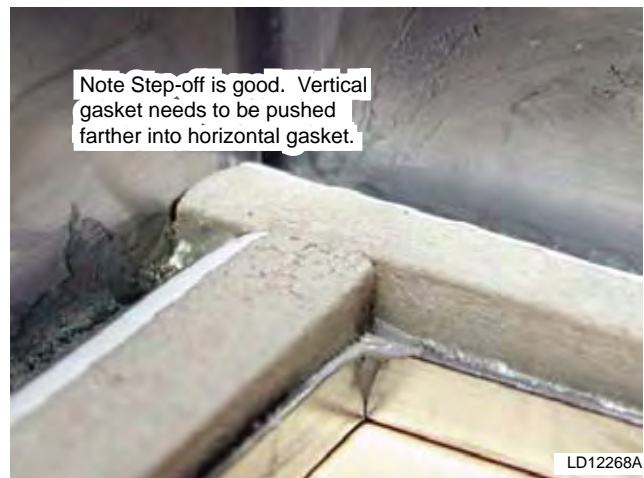
FIG. 5-65 – UNACCEPTABLE BUT JOINT, VERTICAL GASKET NOT PUSHED IN FAR ENOUGH
