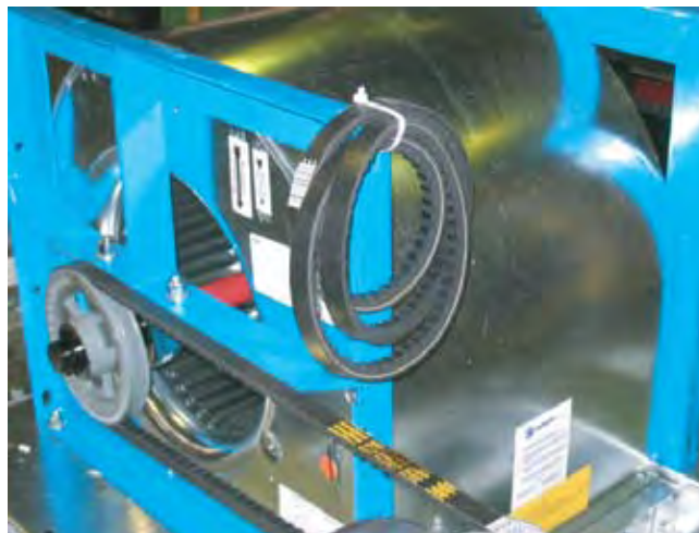
SPARE FAN BELT (Attached to Fan)
